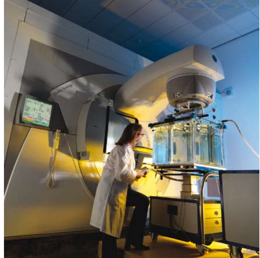
The new Clinical Linac facility at the National Physical Laboratory, funded by DIUS and the Department of Health, is used to calibrate radiotherapy equipment ensuring safe operation
